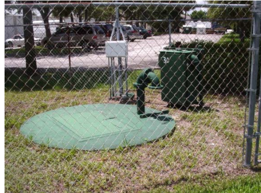
Lift Station Odor and Airborne Bacteria control
